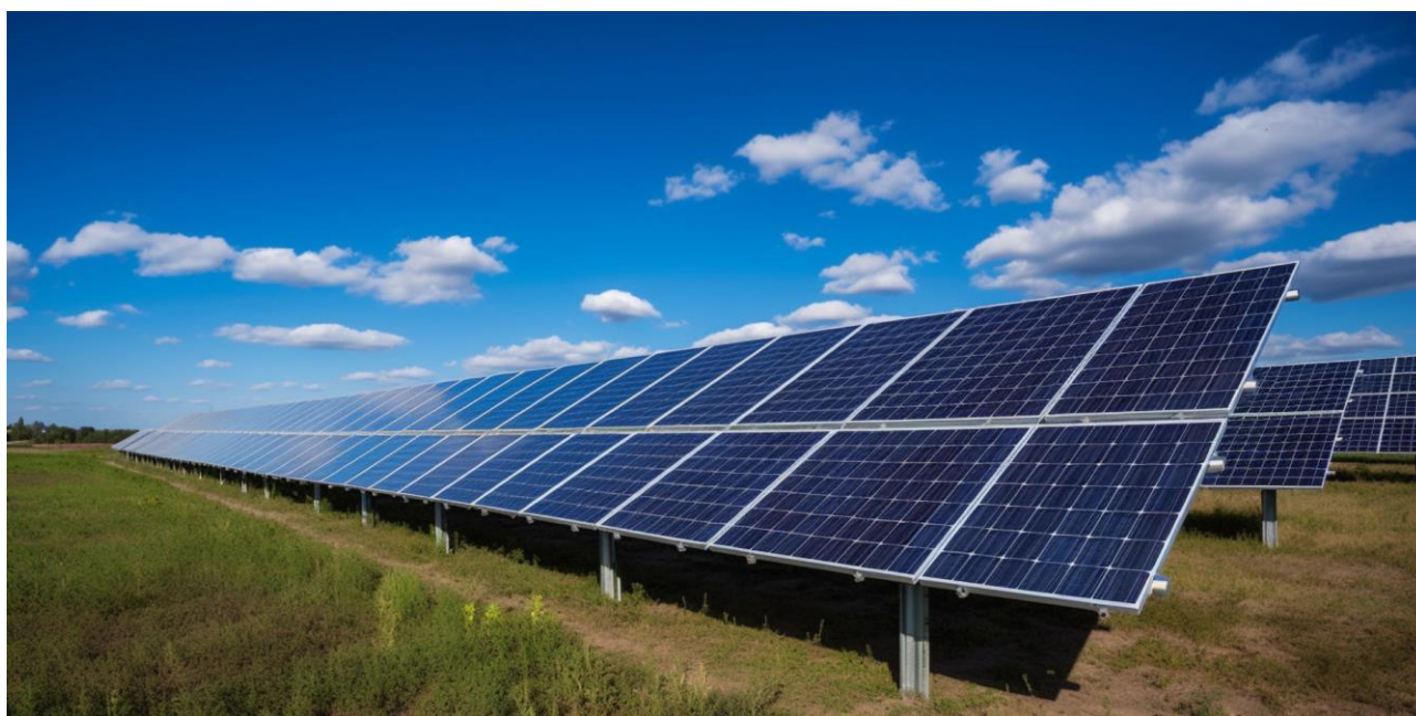
Figure 5.2 Indicative Solar Array and mounting structure
